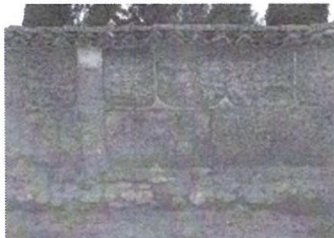
Figure 10. Rammed earth wall with gypsum 'brenças' in Rincón de Ademuz (Valencia), 2015. Photo: Vegas & Mileto
