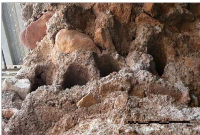
Fig. 18. Imprints of the reinforcement logs for the lintel of the access room (V. Cristini).
