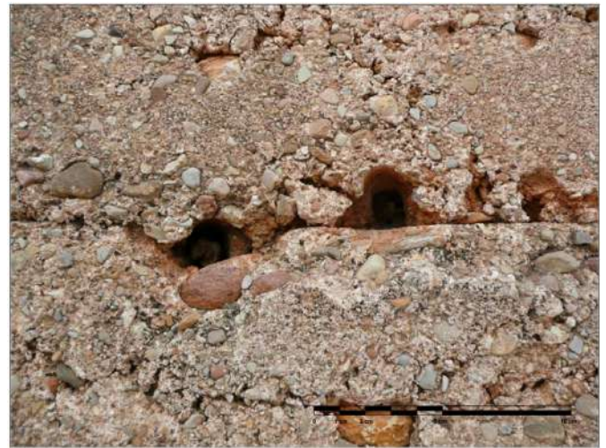
Fig. 3. Putlogs of the formwork inside the walls of Bofilla Tower (C. Mileto and F. Vegas).
