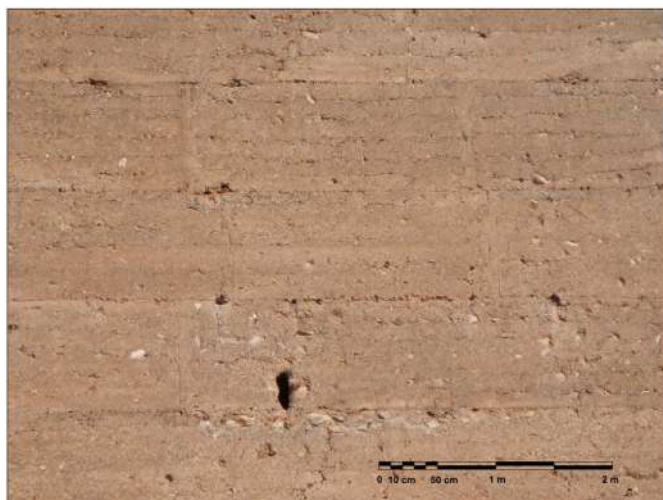
Fig. 4. Imprints of formwork in walls of the Bofilla Tower (C. Mileto and F. Vegas).
