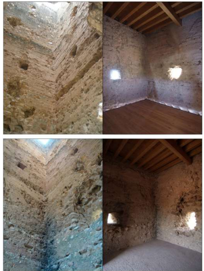
Fig. 21. New floor project, respecting the imprints of original planks (C. Mileto and F. Vegas and T. Baeza).
