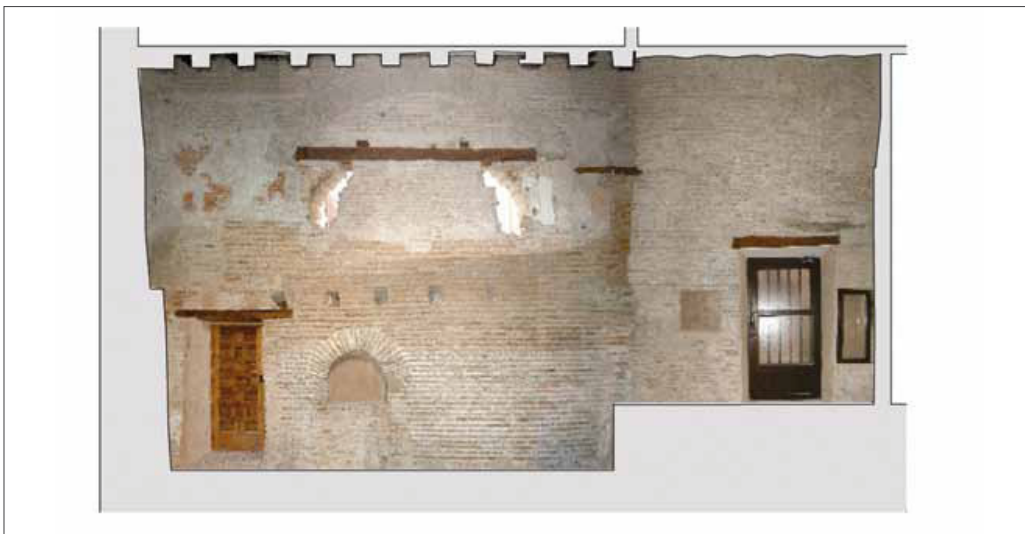
Fig. 3c Antechamber of the Mexuar in the Alhambra (Granada, Spain). Photoplan of elevation no.1 after restoration
