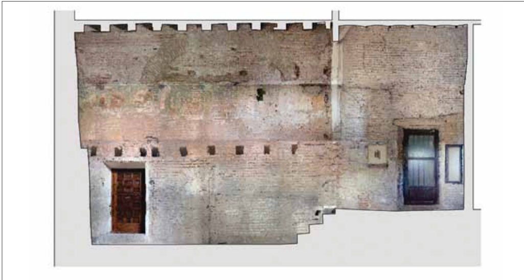
Fig. 3a Antechamber of the Mexuar in the Alhambra (Granada, Spain). Photoplan of elevation no.1 prior to restoration
